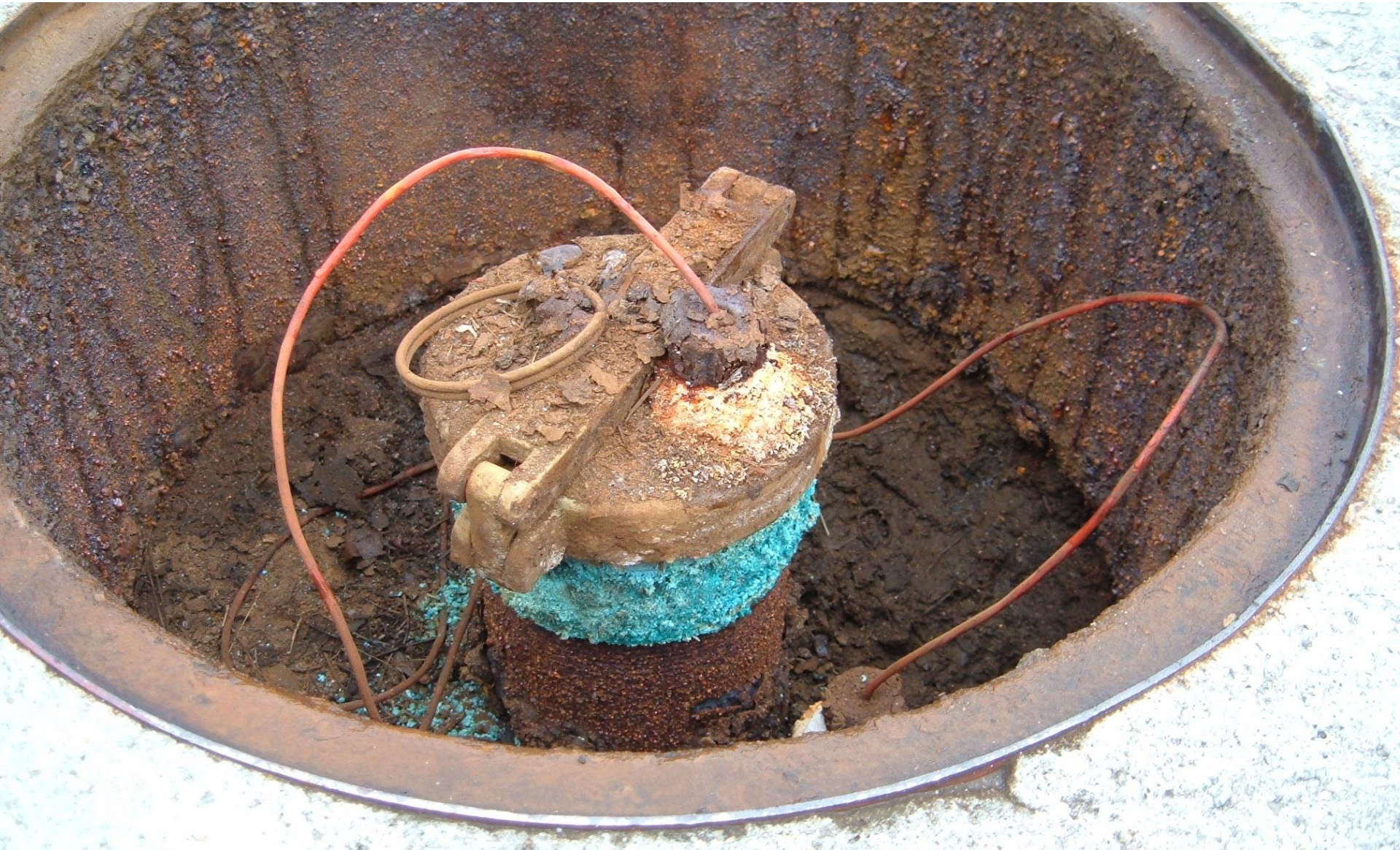
Evidence of vapor leaks
