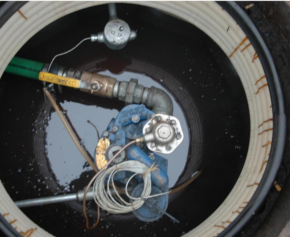
Diesel sump, same facility, Georgetown, South Carolina, November 2011
