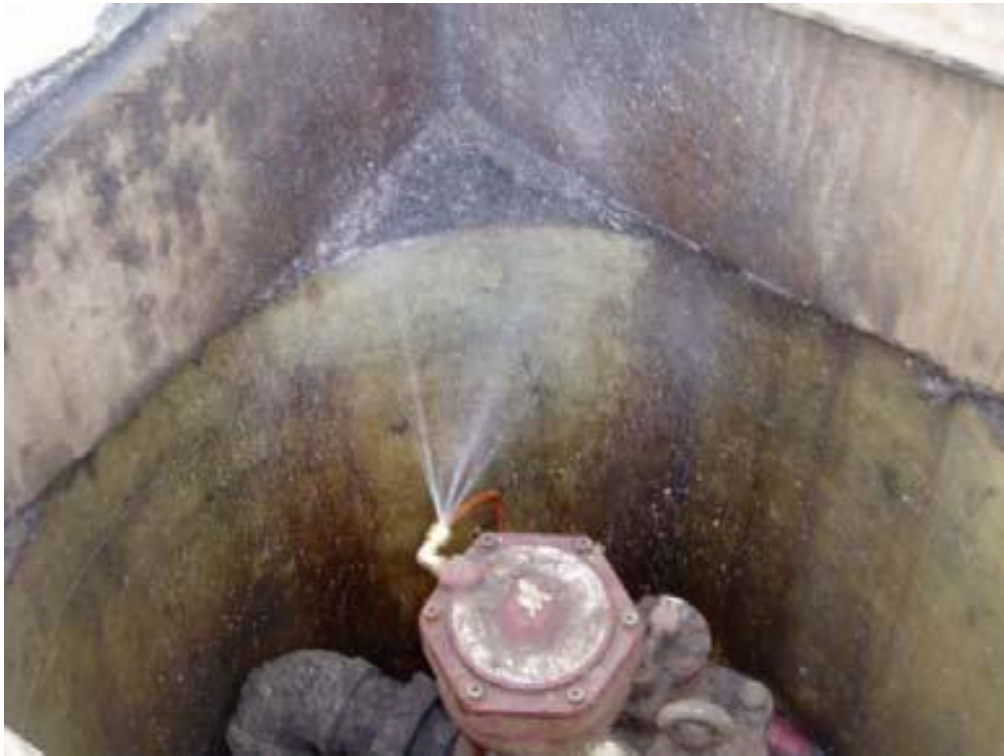
Leaking Line Leak Detectors
